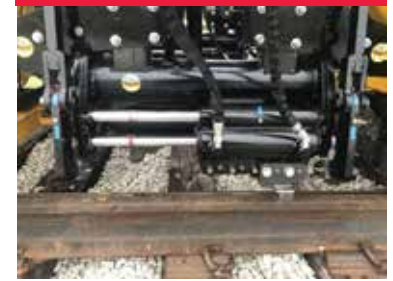
Close up of workhead (Raised position).
